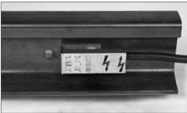
Coverplate mounted on railcontact
